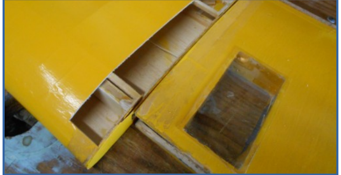
Photo 5: Not only was the end rib on the right panel not connected to the rest of the wing but the plywood itself had delaminated. It appears the struts were doing all the heavy lifting.
