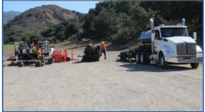
After patching the cracks (mostly) the guys went to work on the reslurrying.
